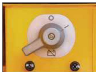
BATTERY DISCONNECT SWITCH
